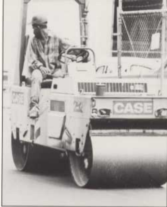
Left: This Case 252 was one of several rollers used on the project. Below: Final paving on a portion of the Winn Dixie project.
