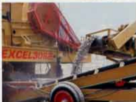
Old pavement is crushed (top) and finished material flows through Dykes Paving & Construction's Excel recycling plant.
