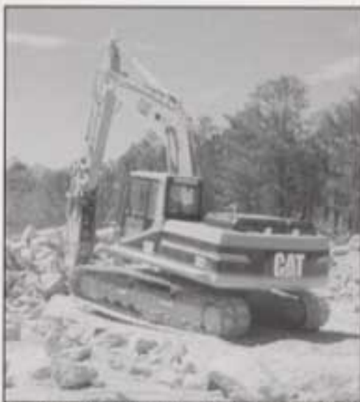
A Cat 322 excavator, equipped with an Okata breaker, prepares concrete for recycling.
